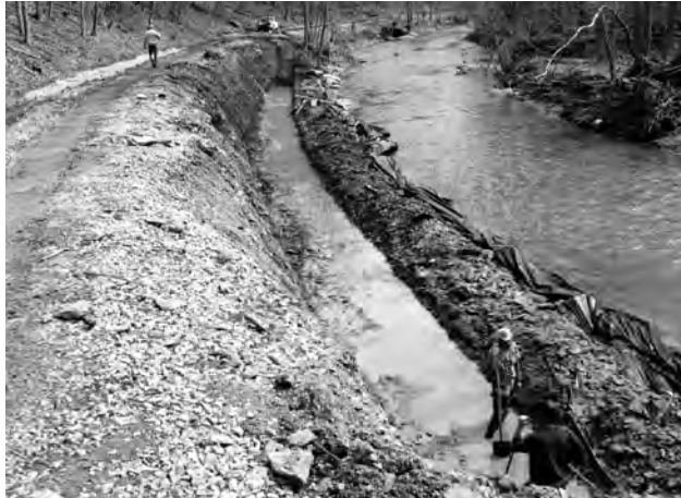
Extensive excavation and a large diversion dike were required so that the footing could be poured for the gabion wall at S-1 (Photo courtesy of Mark Wilson)
