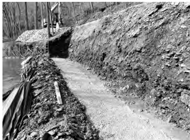
The finished footing, ready to receive the gabion wall at the north end of S-1. (Photo courtesy of Mark Wilson)
