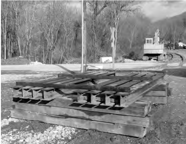
The deck of bridge B-2 was set up on ties south of High Rock Rd. for inspection (Photo courtesy of Craig Sansonetti)
